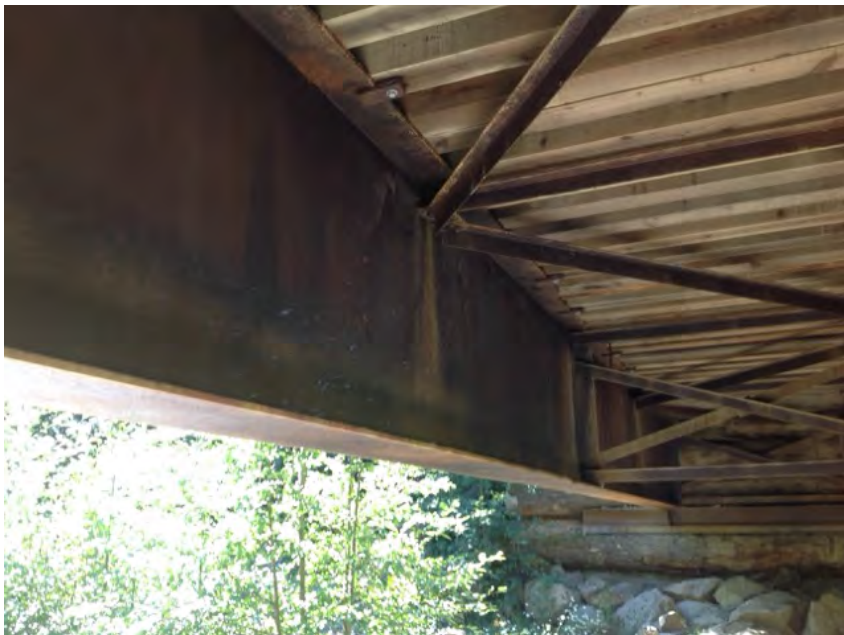
corrosion on upstream girder
