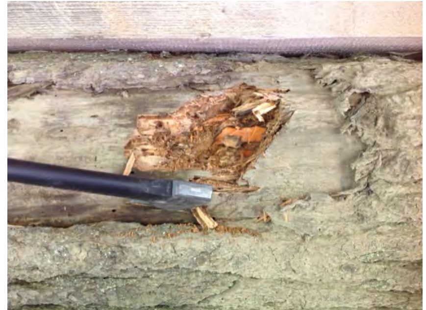
up to 60mm sap rot on top crib logs - no signs of crushing
